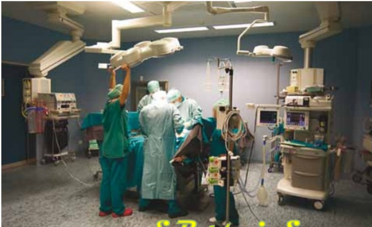
Group 2 medical locations, operating room
